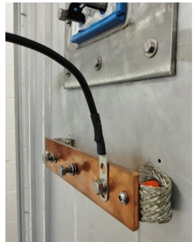
Bonding between bar and cabinet wall via two large flat braids, on both extremities of the bar.
