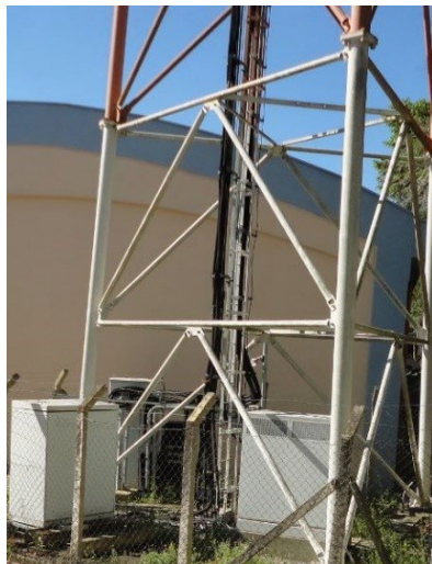
Figure 7b: Same site as in fig. 7a, where a number of antenna cables go to telecommunications equipment in outdoor cabinets installed at tower foot.
