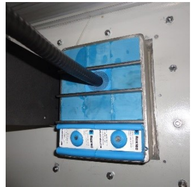
Cable entrance via isolating ROXTEC modules. Viewed from inside.
