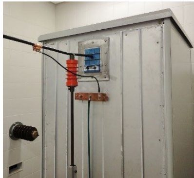
Connection to earth via earthing kit, external bar and external 35 mm 2 conductor. See also fig. 12.
