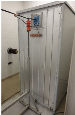
Connection to earth via earthing kit to the external bar, which is bonded to the cabinet wall.
