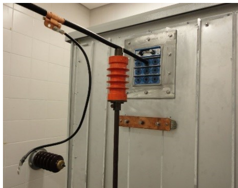
Cable bonding to cabinet via ROXTEC BG B. The earthing kit appears hanging loose in the picture.
